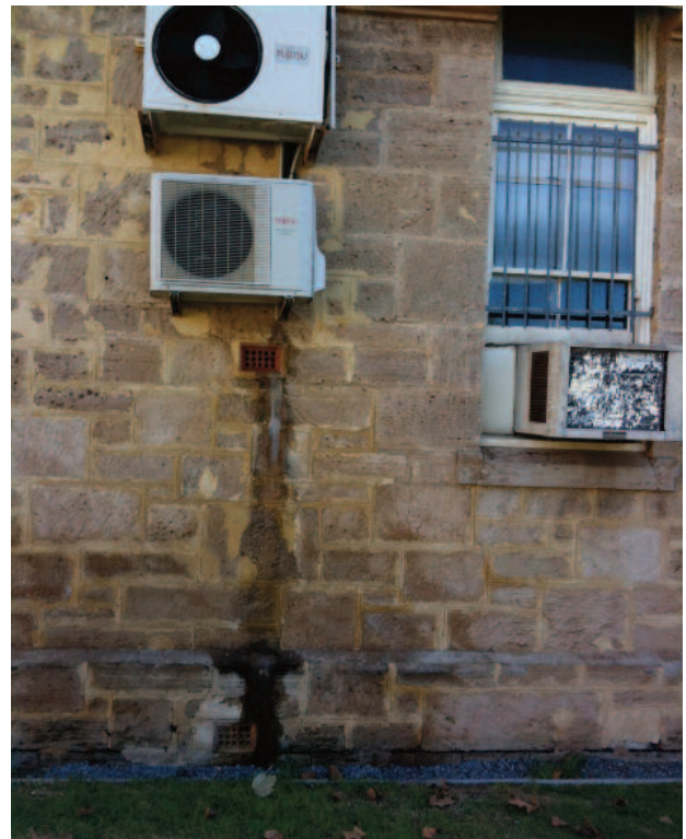
Above: Inappropriate airconditioners and rising and falling damp scar the highly significant 1854 boys' school.
