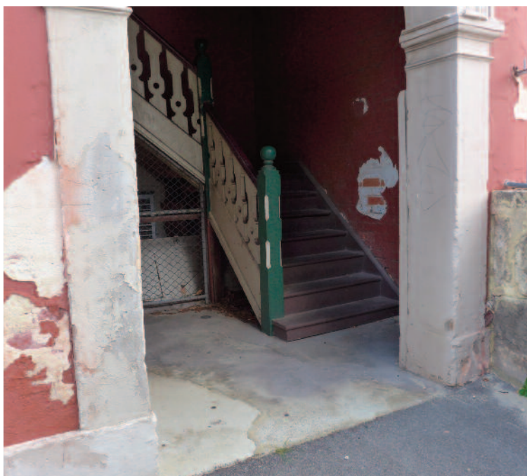
Above: A shocking lack of maintenance by Fremantle Council is evident.
