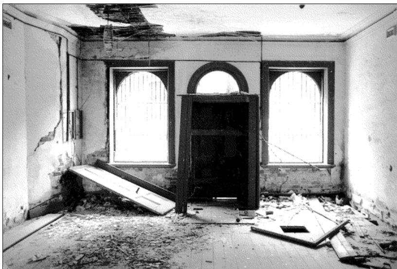
Figure 5: Debris in the front room of the former Residence in 1986
