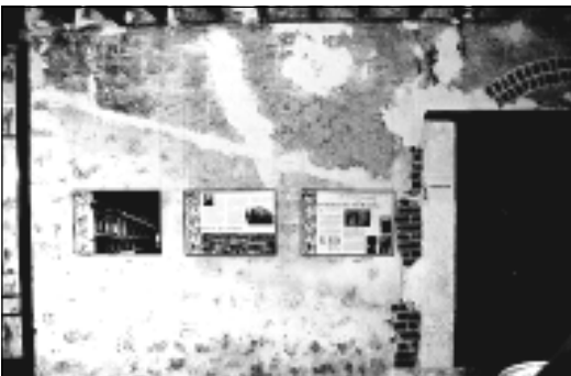
Figure 21: The position of metal ties in the wall and the concrete anchor against the door jam can clearly be seen. Also note the brick quoins and arch to the former doorway
