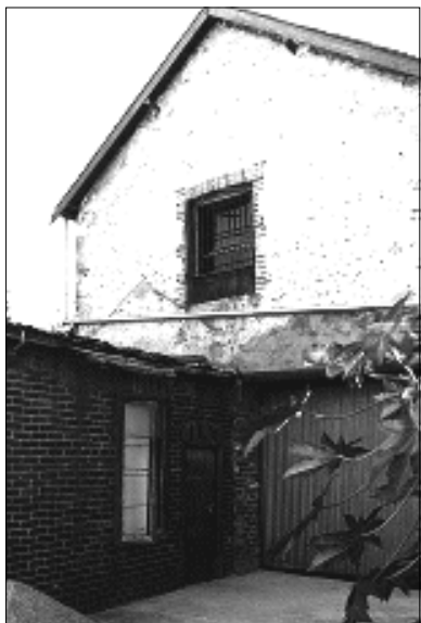
Figure 14: The flashing line of the former Stable roof was evident on the rear wall of the warehouse
