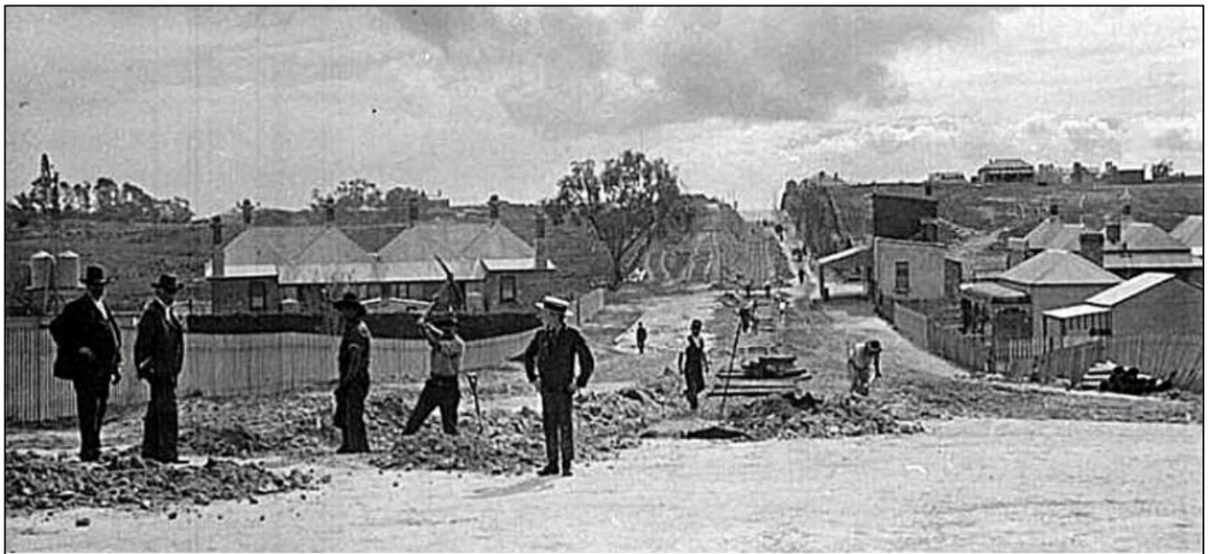
1 st August 1905. Tramway track under construction. Looking north on East St. from High St. with the corner shop on Holland St. in the middle ground. The earth removed from the East and Ellen St. cuttings was carried by horse-drawn drays and used to reclaim Fremantle Esplanade. Fremantle History Centre LH002433
