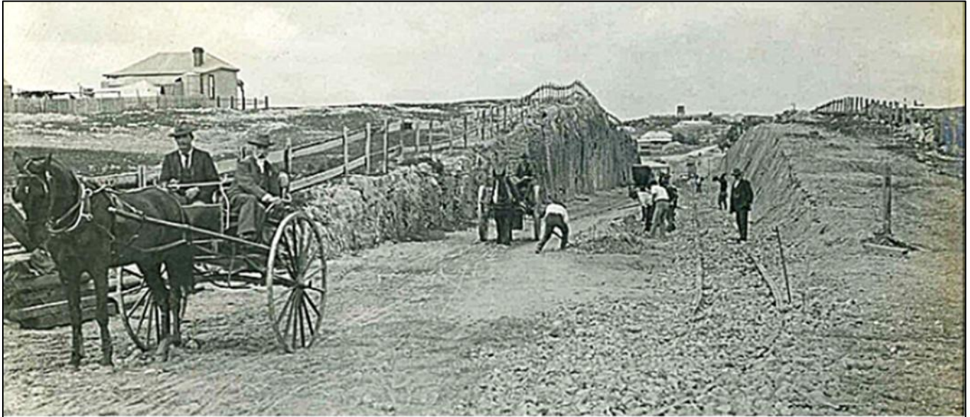
28 th July 1905. Tram cutting at East Street, corner of Marmion Street, Fremantle. Workmen preparing the road for laying tram tracks. Fremantle History Centre EF0019
