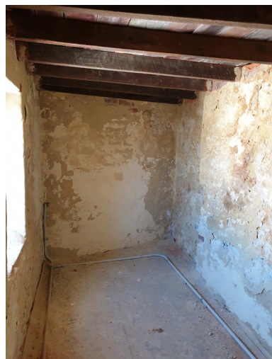
Images 3-5: The southern, central and northern rooms of the 1844 upstairs Gaoler's quarters (photos by author).
